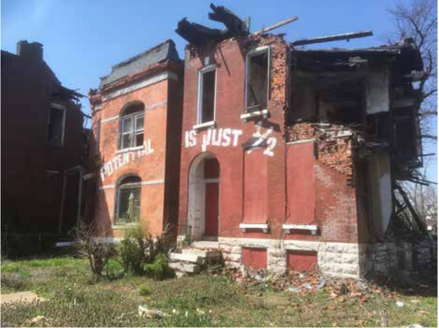
Vacant houses on Cass Avenue in St. Louis. Photograph by the author, 2018.
