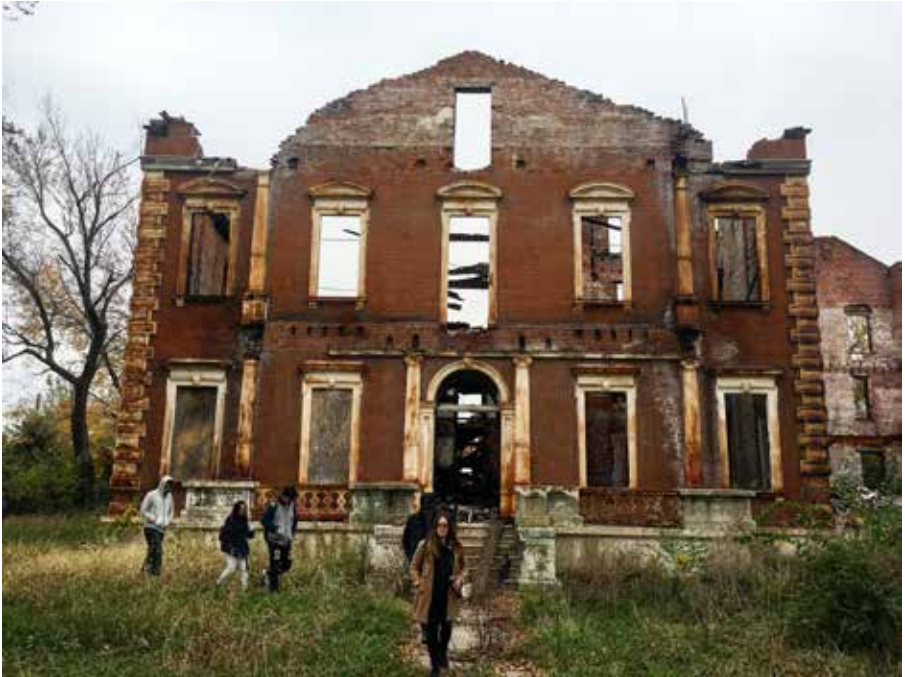
The James Clemens House in north city St. Louis, destroyed by fire in 2017. Photograph by the author, 2017.
